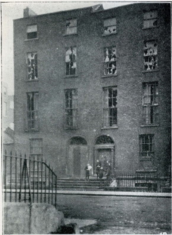
Dilapidated houses, 30 and 31 Grenville Street.
